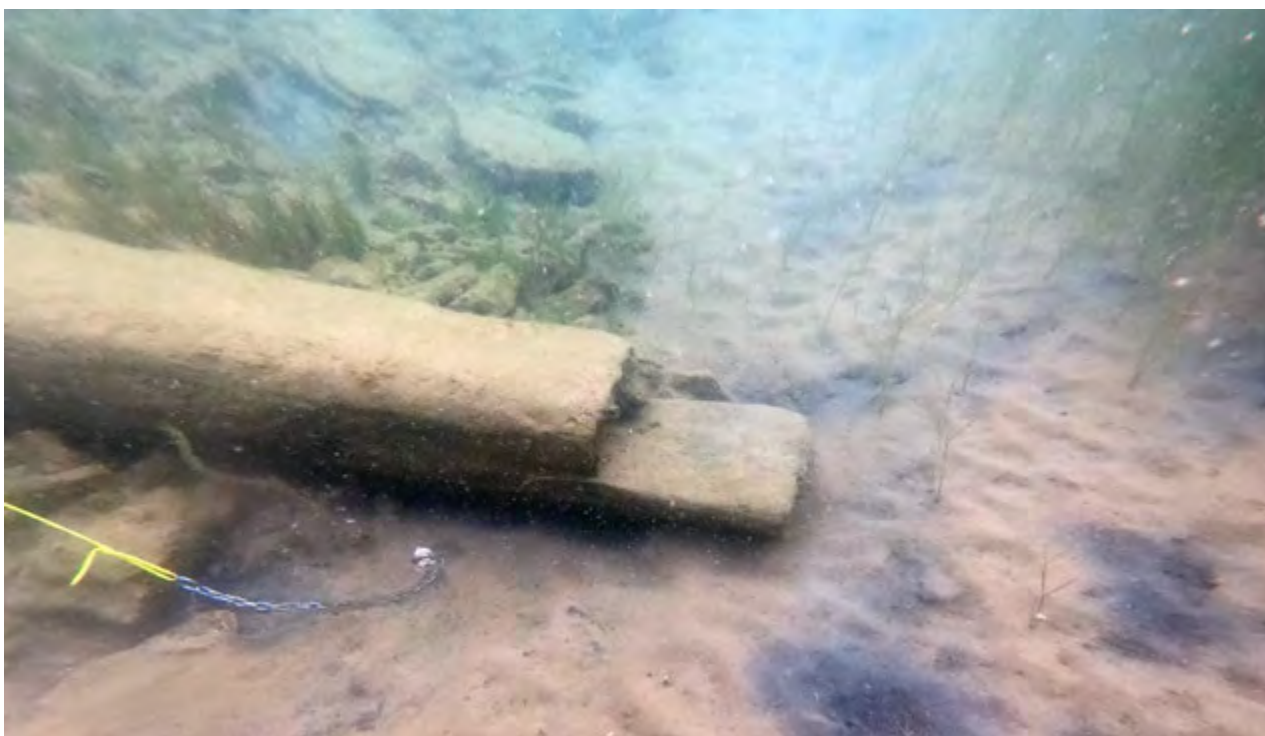
Figure 84: Half-lap notching of a crib timber at Higgins Pier.
