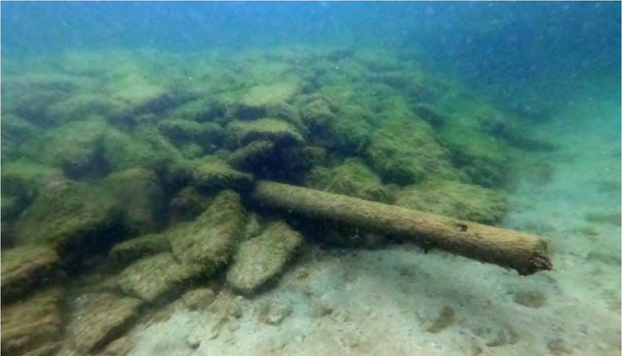
Figure 108: Timber protrudes from the sloping side of a collapsed crib.
