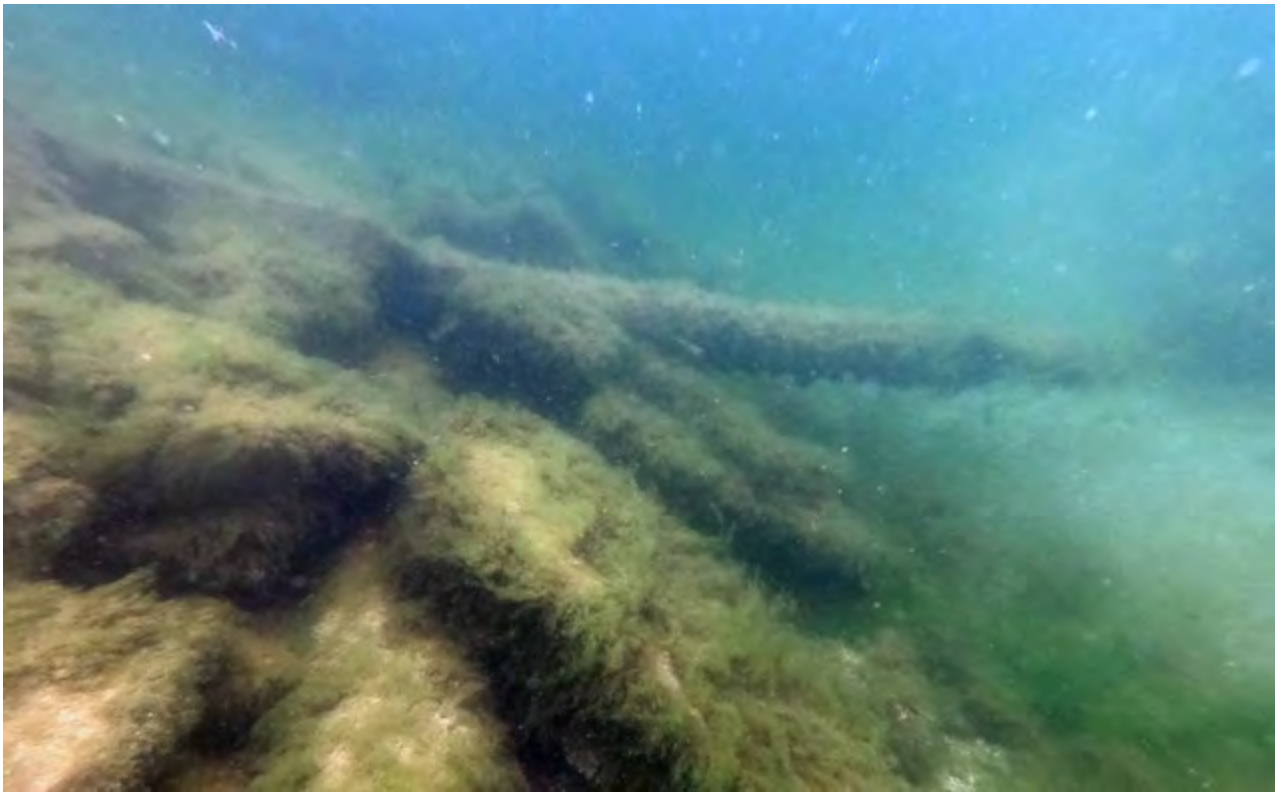
Figure 140: A timber protrudes from cribbing stone at Torstenson's Pier.
